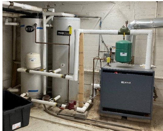
Indirect DHW system, with two tanks connected to a boiler
